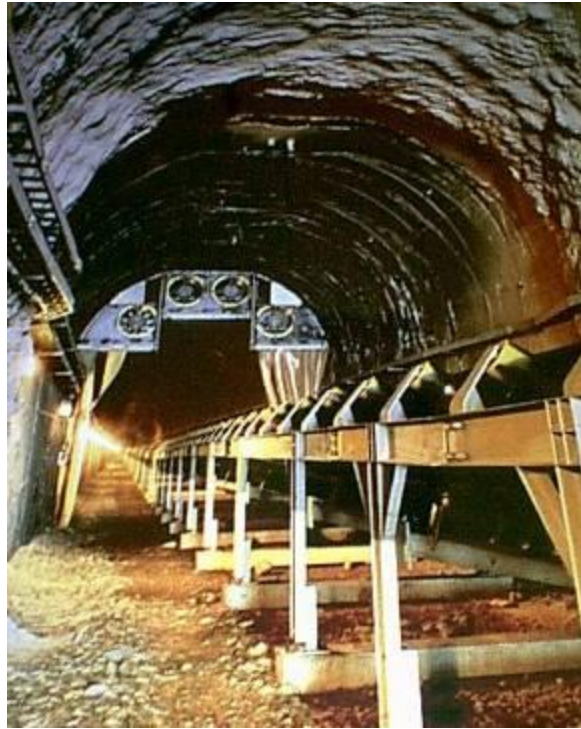
Fig. 6 C-6 Conveyor in the tunnel
