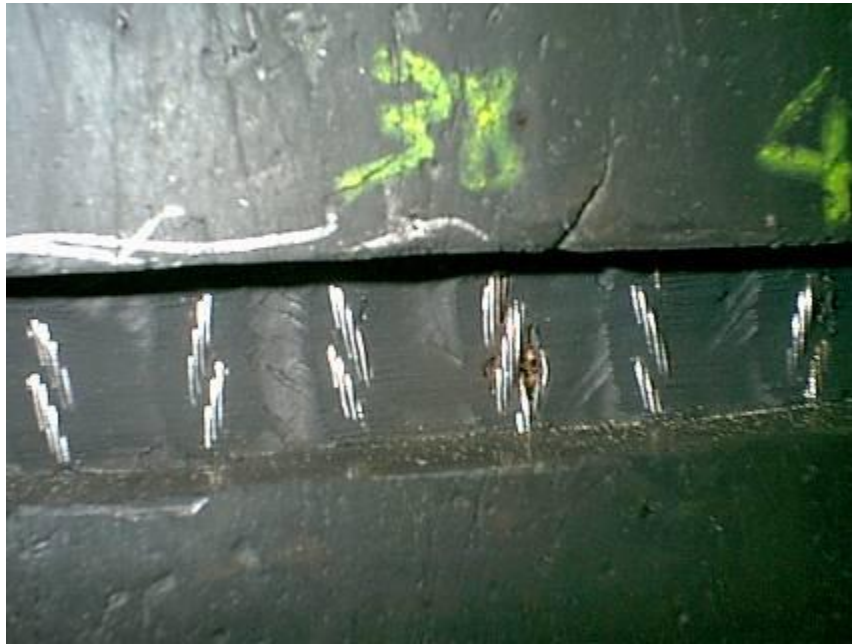
Fig. 16 Example of cord corrosion initiated from impact damage
