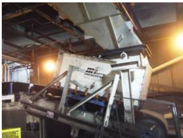
FIGURE 3 Engineered Chutes as Installed on the Bunker Feed Conveyors at Meramec Power Plant.
