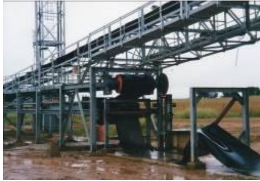
Illustration 7 – Uphill belt conveyor at Middelburg Mining Services with BSFH350 MS brake and two-stage hydraulic system
