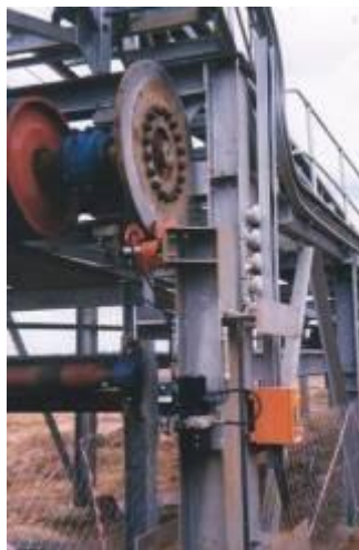
Illustration 8 – BSFH350 MS brake and two-stage hydraulic system installed at Middelburg Mining Services
