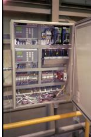
Illustration 24 - The SOBO control system with two SOBO controllers and battery power backup
