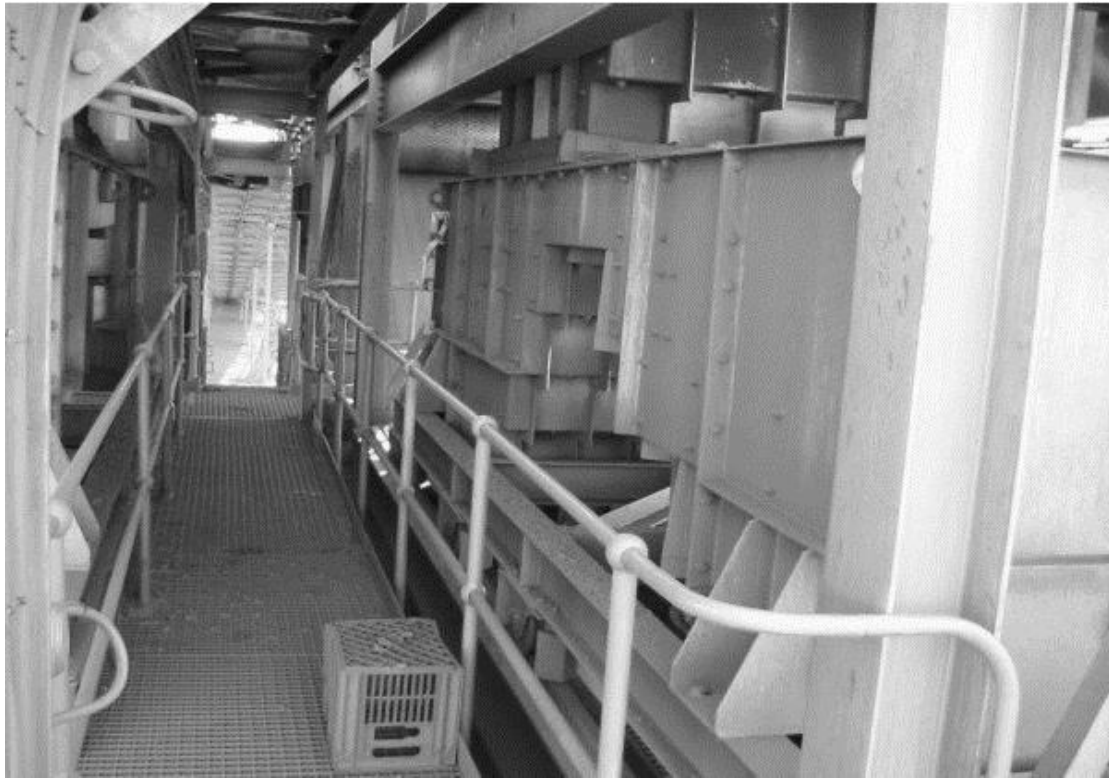
Figure 2.4 – Typical Diverter Chute
