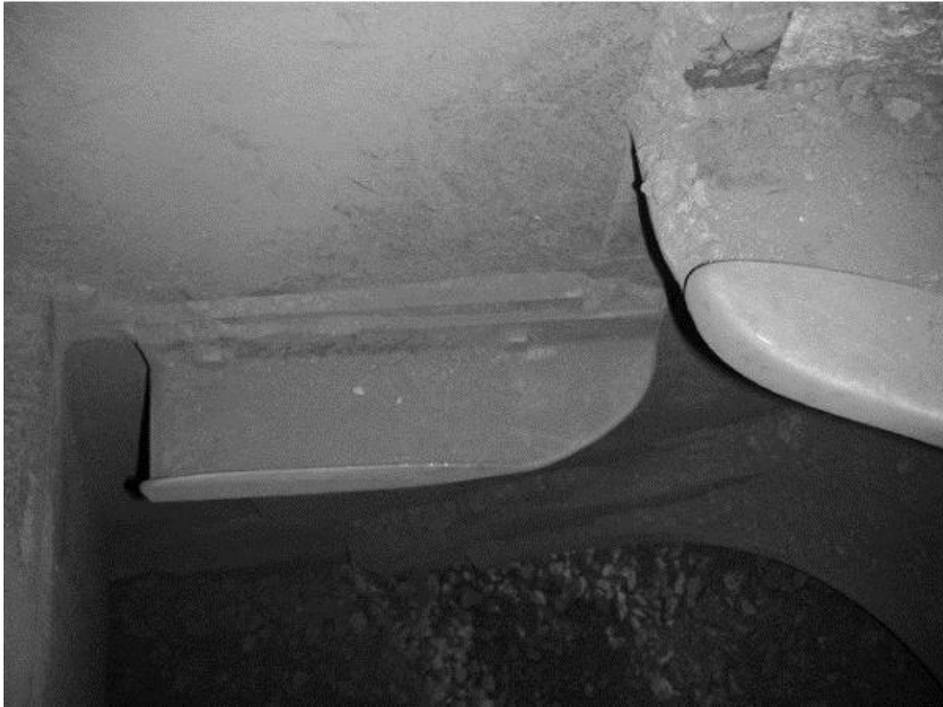
Figure 5-4 – Wear Caused by free fall of ore
