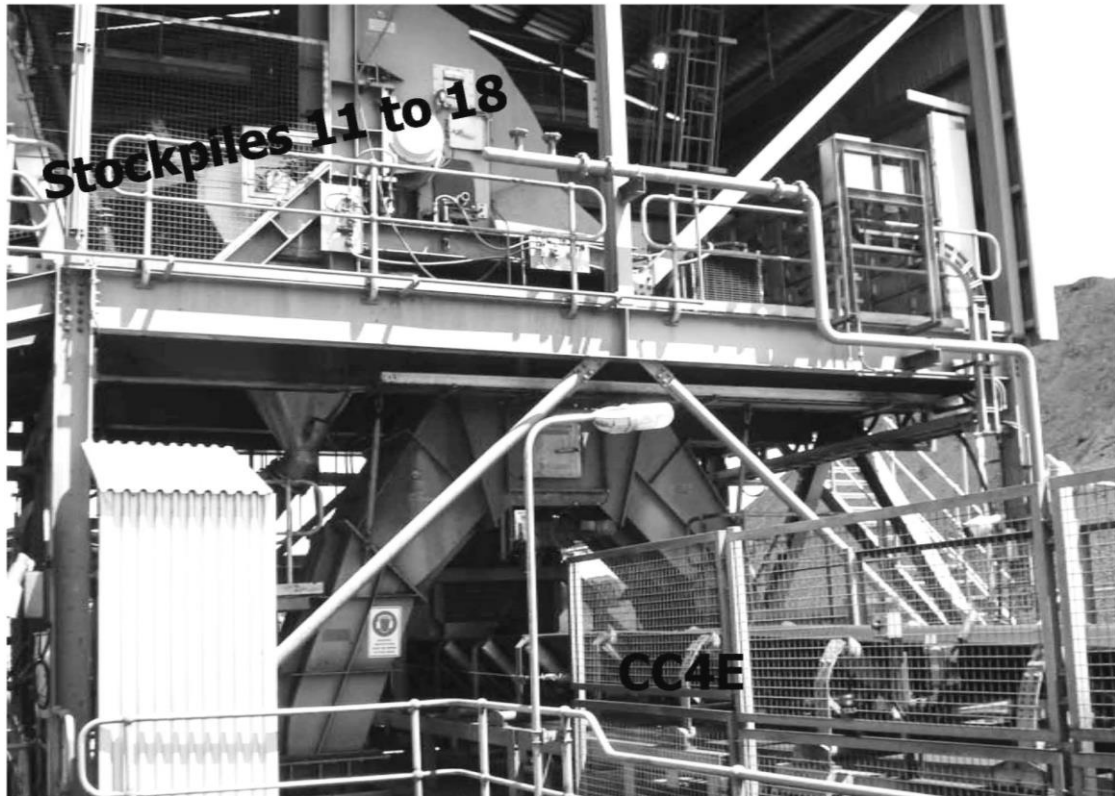
Figure 16. Typical third shipping stream CC4E transfer tower
