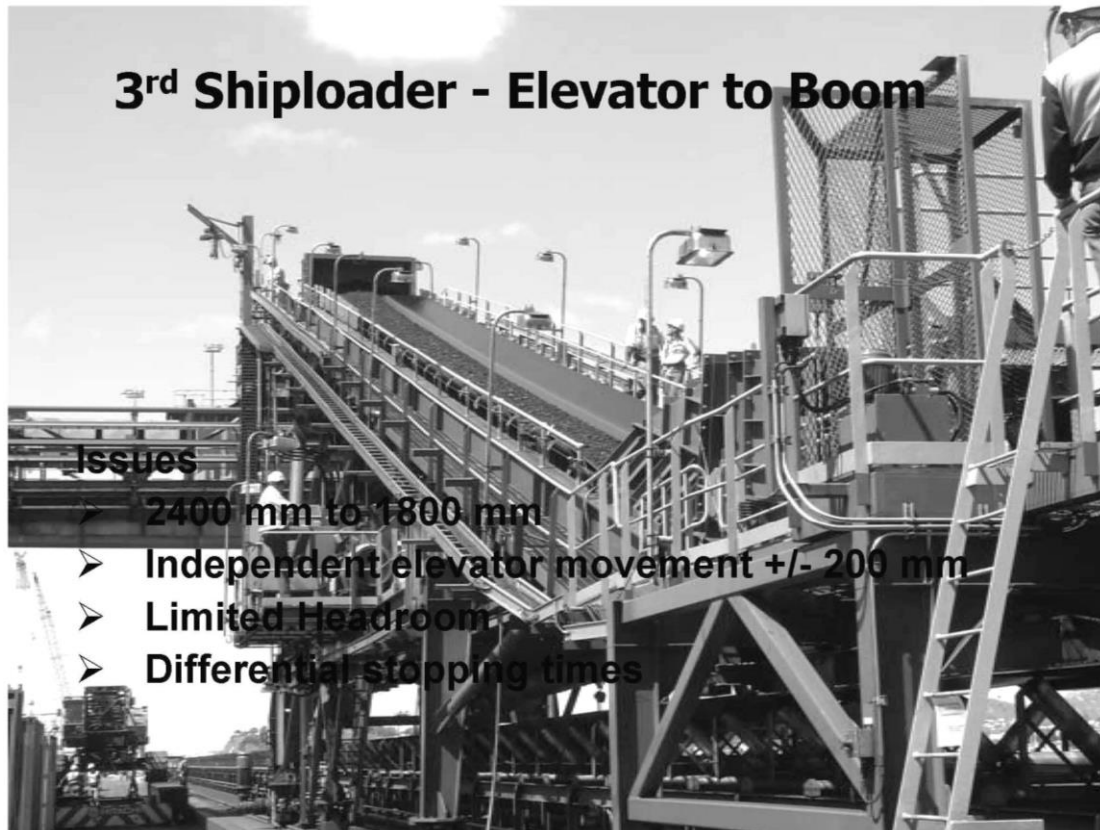
Figure 17. Third shiploader, elevator to boom
