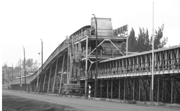
Figure 4. CV623 New stockyard spine conveyor transfer
