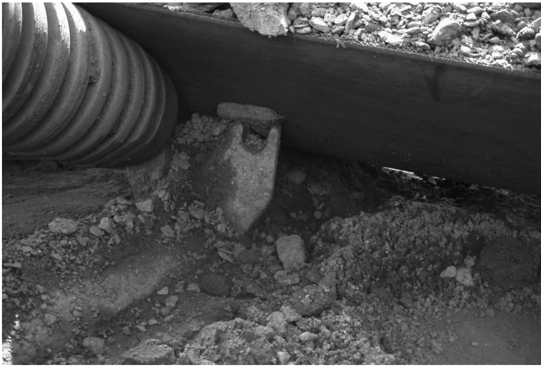
Figure 10. No maintenance, totally overloaded
