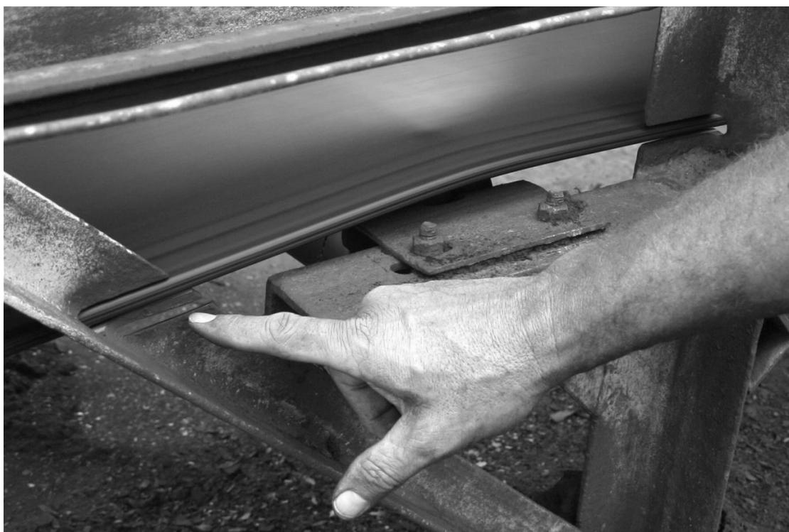
Figure 6. A poorly tracked belt led to serious structural damage
