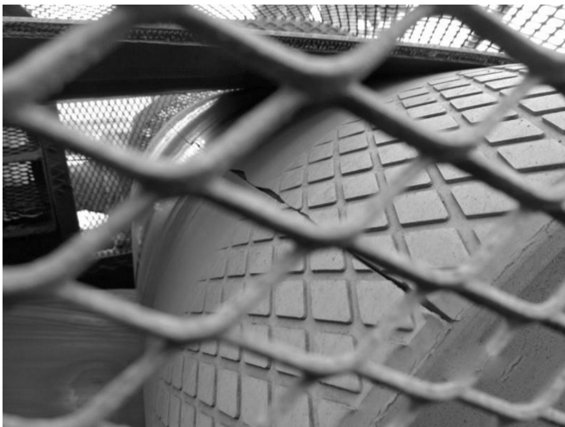
Figure 5. Severely damaged pulley lagging
