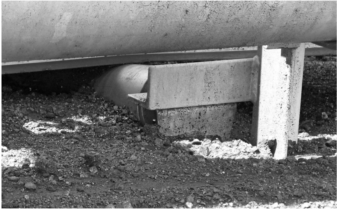
Figure 7. Return idler buried and cannot rotate or be replaced due to tripper discharge
