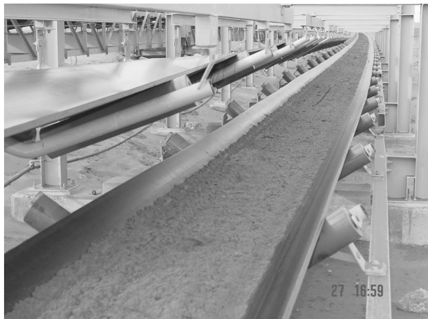
Figure 3. Relocated mine end tripper/drive
