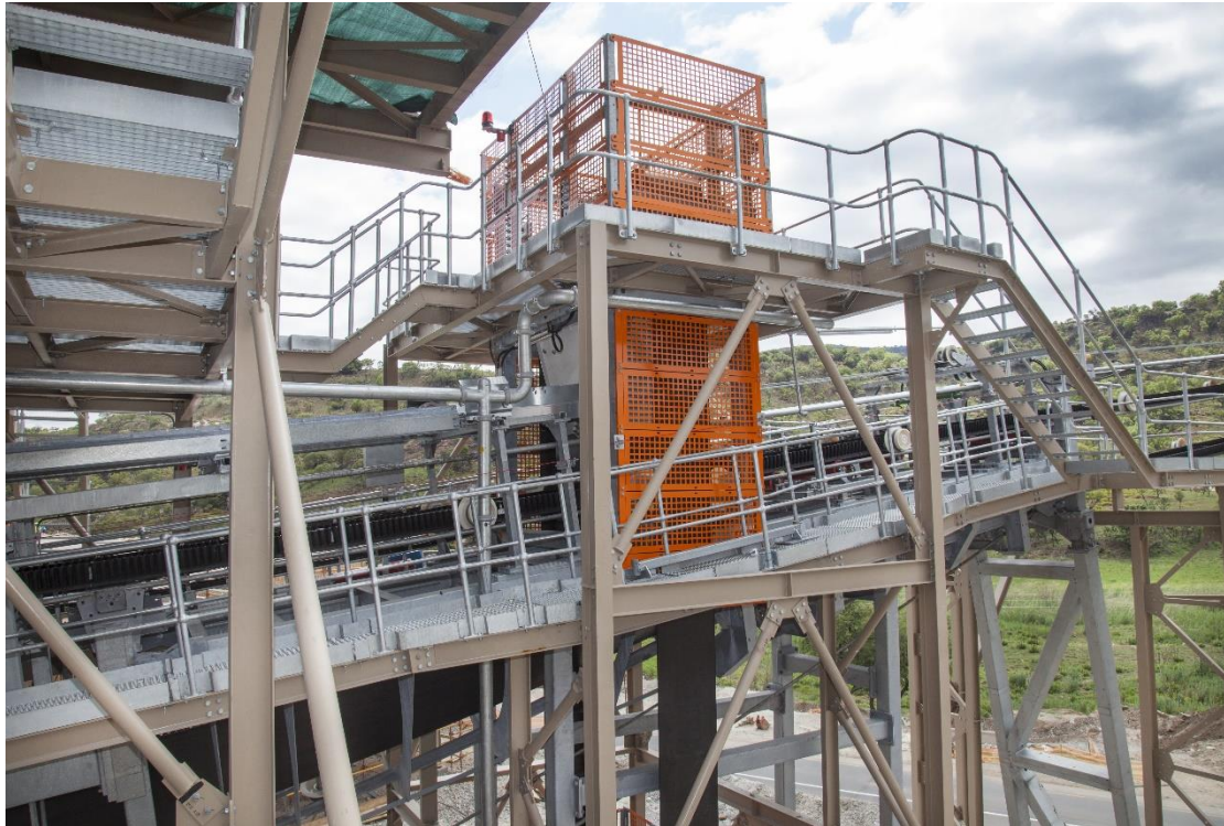
Figure 10: Vertical spillage conveyor circling the RopeCon after the loading points.
