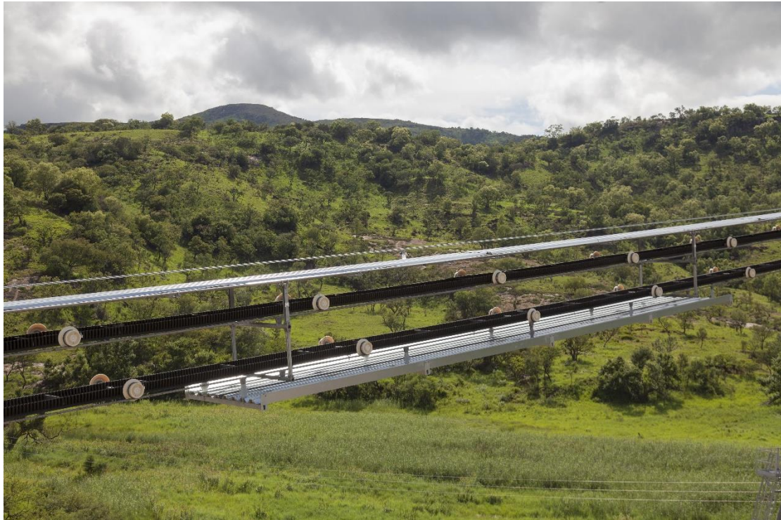
Figure 30: Covering underneath the RopeCon where it crosses a road.
