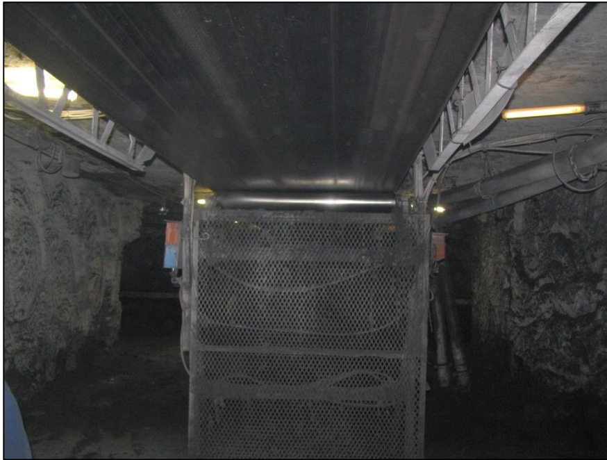
Figure 8. Image showing the lack of guarding at the belt bridge.
