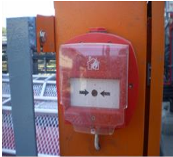
Figure 12. Emergency activation alarm
