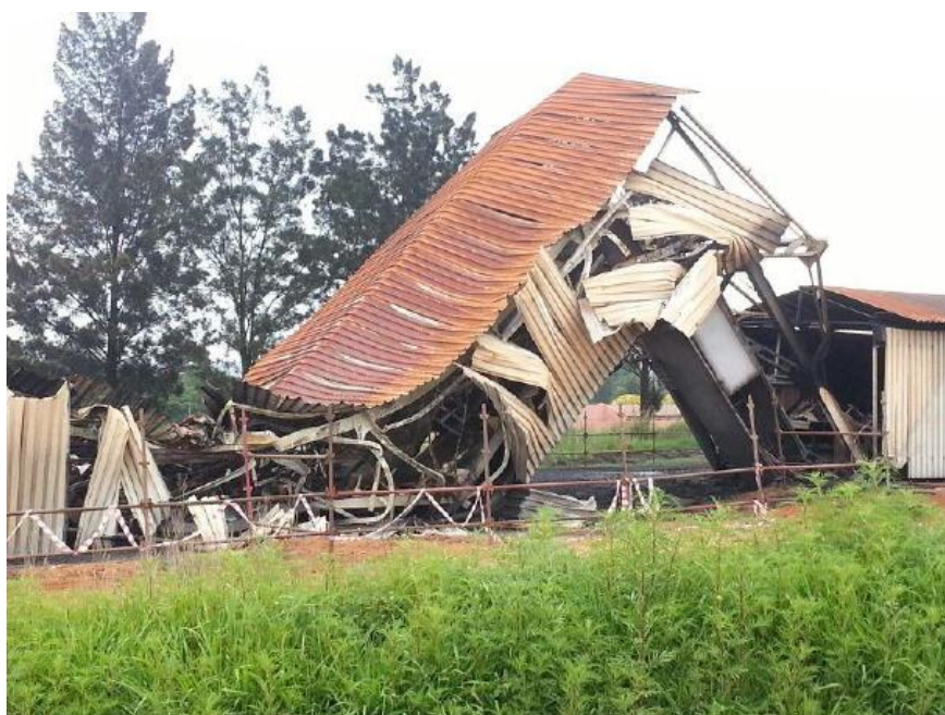
Figure 3. Damage to conveyor belt structure after Duva Power Station fire
