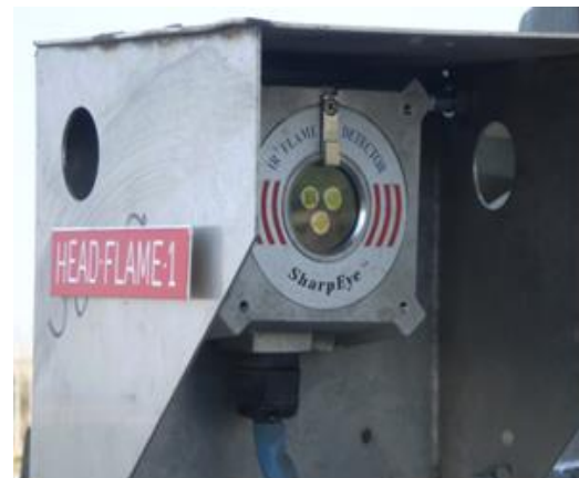
Figure 10. Sounds an alarm and activates the suppression system upon any detection of a flame
